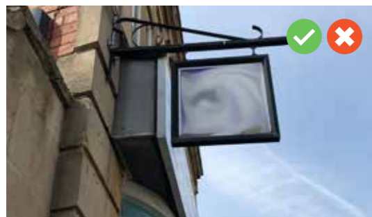
Figure 33. Hanging sign is well positioned but projecting box fascia sign detracts from building character
