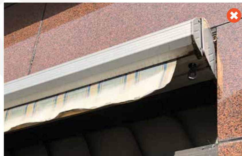
Figure 47. Blind box not well integrated with shopfront
