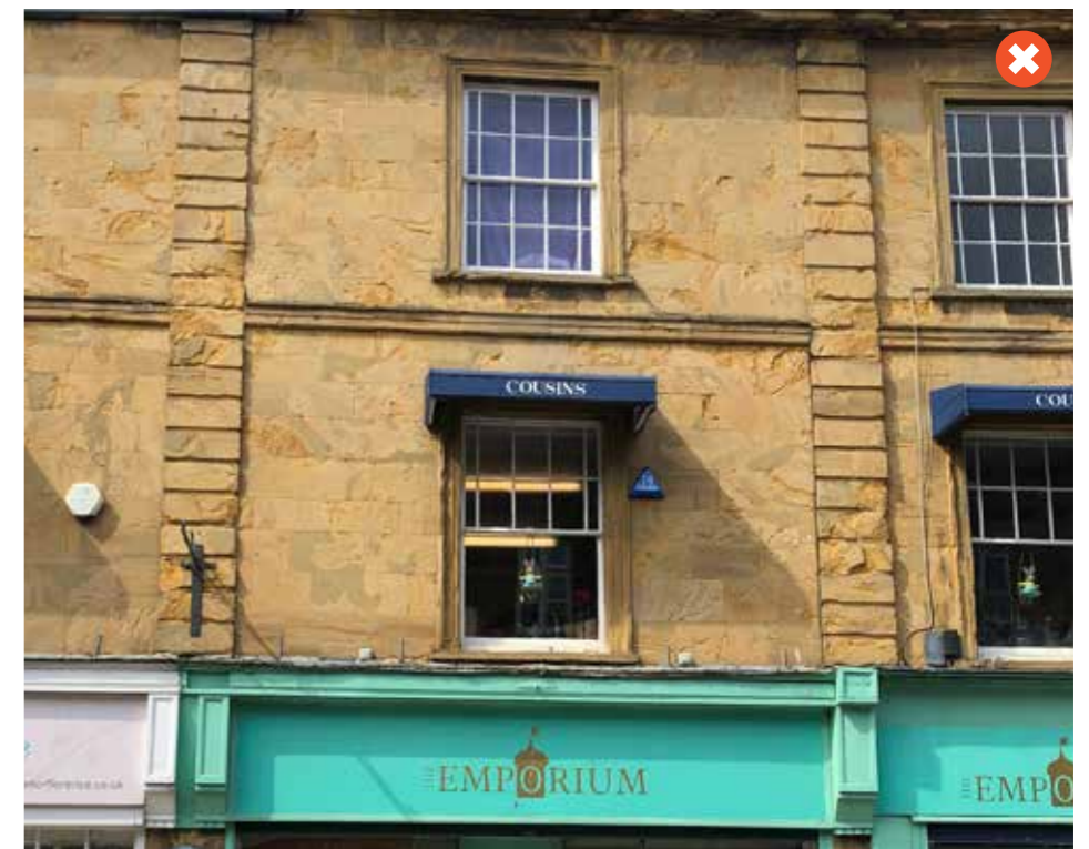
Figure 54. Alarm boxes haphazardly positioned on facade
