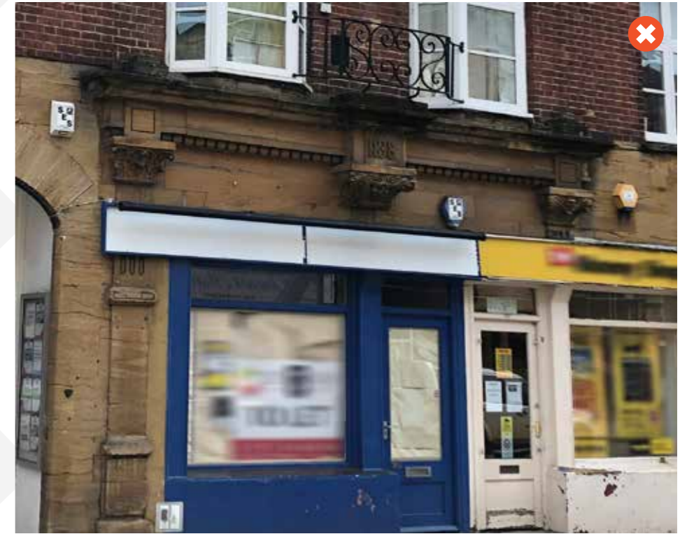
Figure 51. Alarm boxes haphazardly positioned on facade
